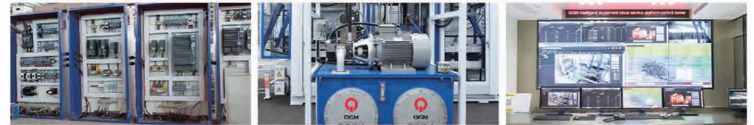
SIEMENS Control System
