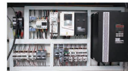
SIEMENS Control System
