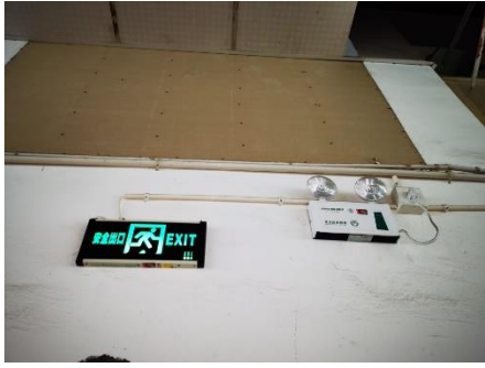
Emergency light and exit sign
