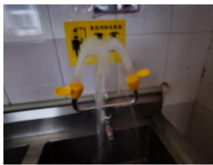
Eye washing facility
