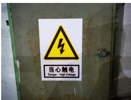
Switch box with warning sign
