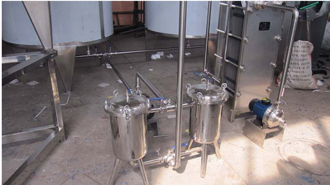
Duplex Filtering Unit
