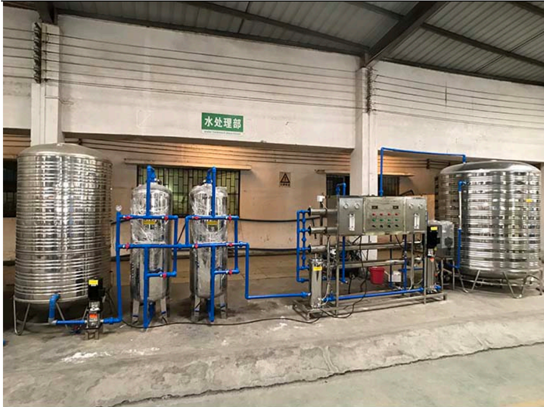
2000LPH RO Water Treatment System
