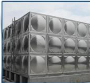
Stainless Steel Tank
