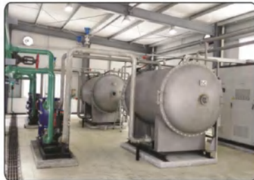
FEIXIAN SHANGYUAN THERMAL POWER PLANT
