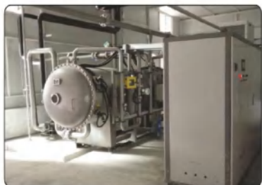
Kenli Petrochemical sewage treatment plant
