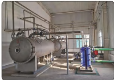
CHIPING SEWAGE TREATMENT PLANT, BEIKONG WATER GROUP
