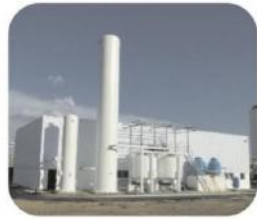
THE AIR SOURCE SYSTEM SUPPLIES AIR
