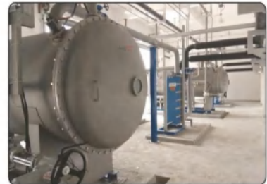
NINGBO ZHONGHUA PAPER WASTEWATER TREATMENT
