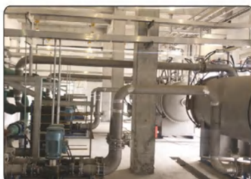
Shanghang County second sewage treatment plant
