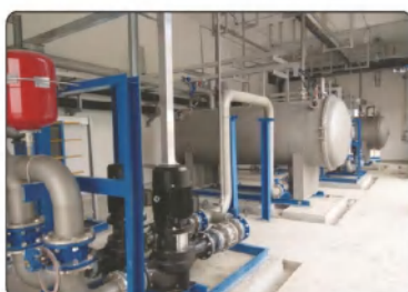
Aksu Textile Industrial City sewage treatment plant
