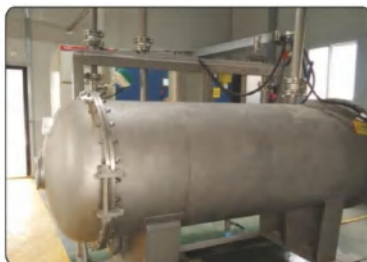
Dongguang County sewage treatment plant
