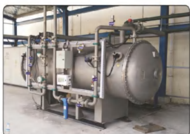
Foshan Nanhai Xinlong Sewage Treatment plant
