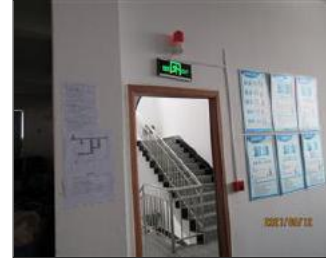
Photo of fire safety equipment 2. Emergency Light. Safety Exit Sign. Fire alarm.JPG
