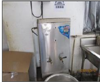
Photo of the sanitary facilities Drinking water.JPG
