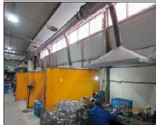
Photo of the inside of the main production hall 1. Welding.JPG
