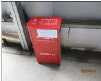
Photo of fire safety equipment 3. Fire extinguishers.JPG
