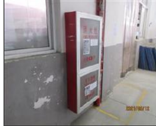
Photo of fire safety equipment 1. Fire extinguishers. Fire hydrant.JPG
