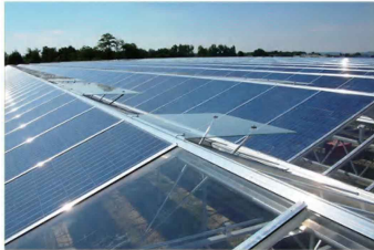
Photovoltaic Power Generation System
