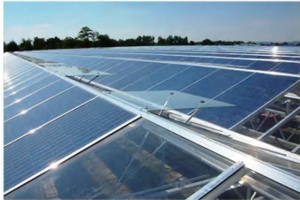
Photovoltaic Power Generation System
